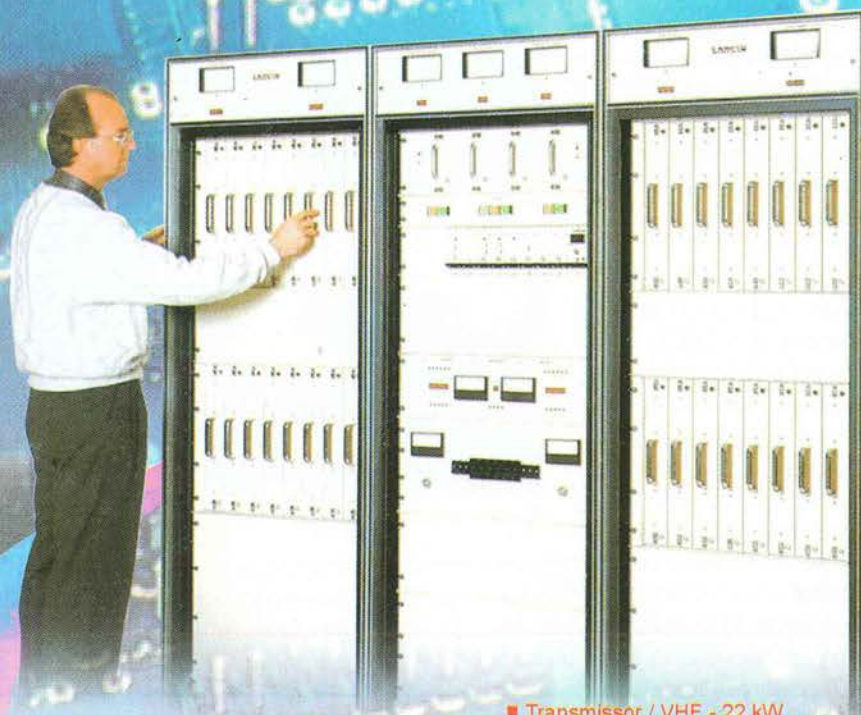
■ Transmissor / VHF - 22 kW
